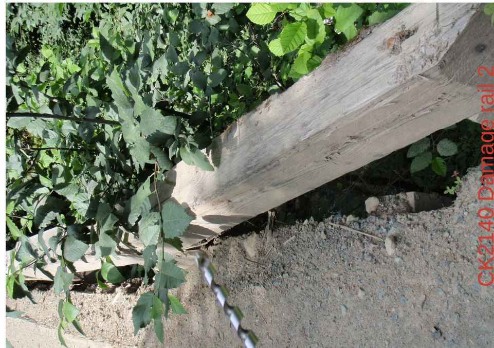
CK2140 Damage rail 3
