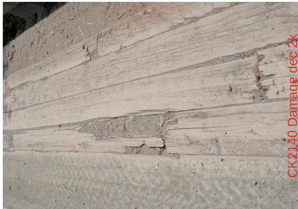
CK2140 Damage deck
